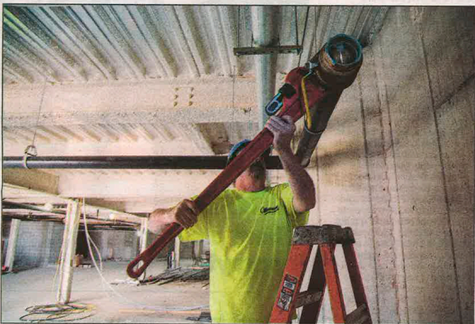
A licensed master plumber at work. The amendment drew praise from the local plumbers union.
